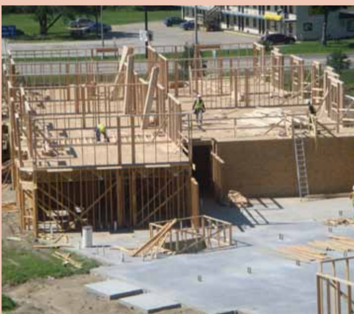
After approximately 4 years of planning, the build of Silveridge Assisted Living began in 2010.
